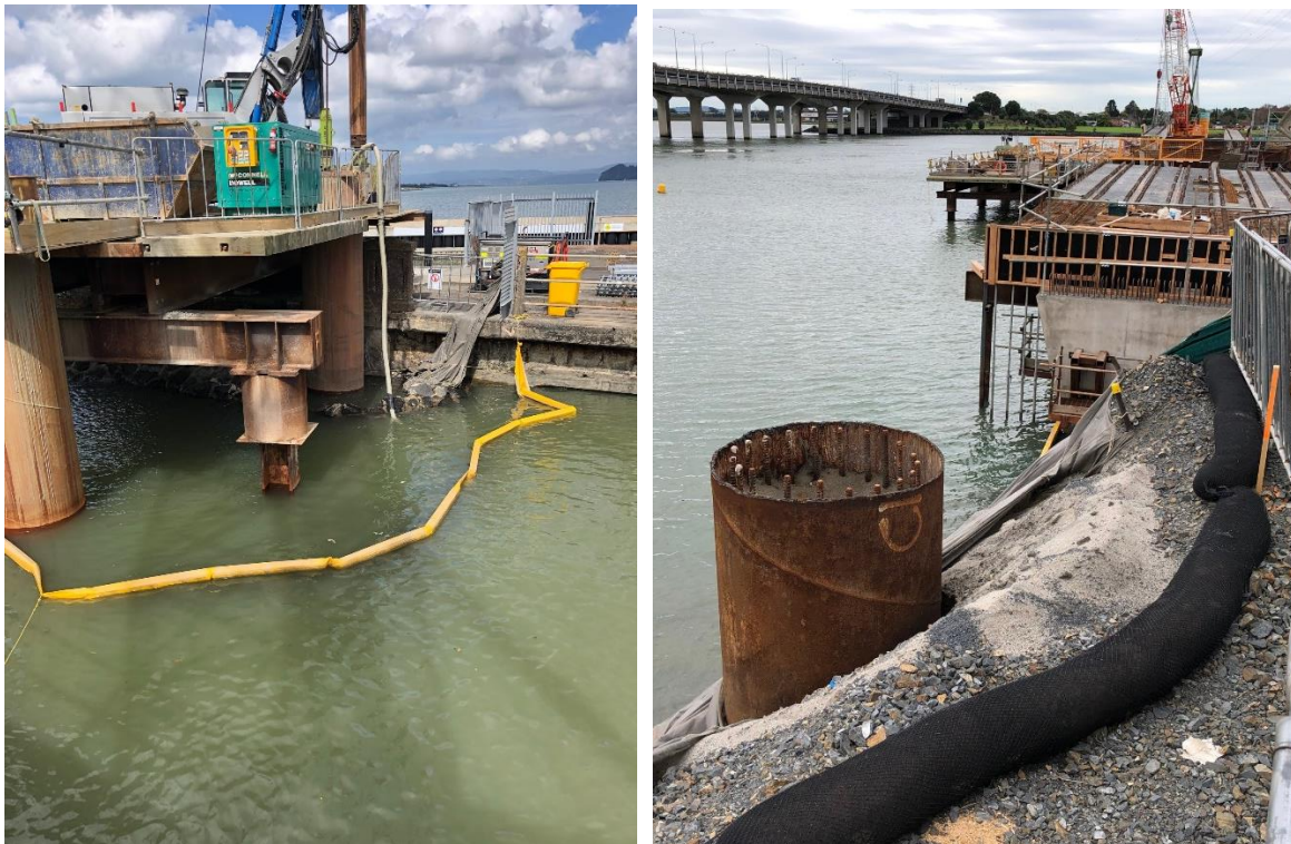
Figure 3 – Examples of silt curtain & silt socks used on a marine piling project
