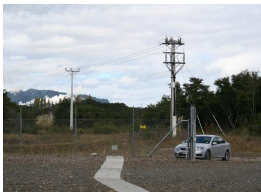
Transmission lines distribute electricity from the power plant to homes and businesses.
